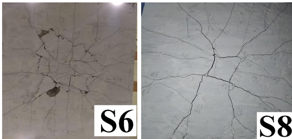
Fig (9): The Crack Patterns for Group 3(c)
